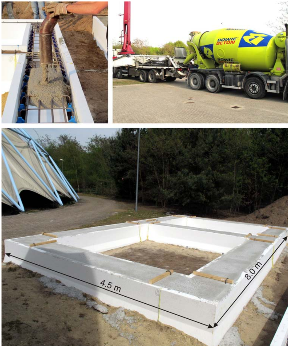
Fig. 6 Cast foundation beam (lower picture) and placing of the SCC (upper pictures)
